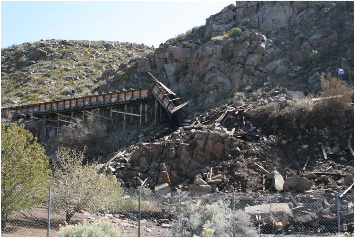
Figure 44 Rock fall damage to water flume.
