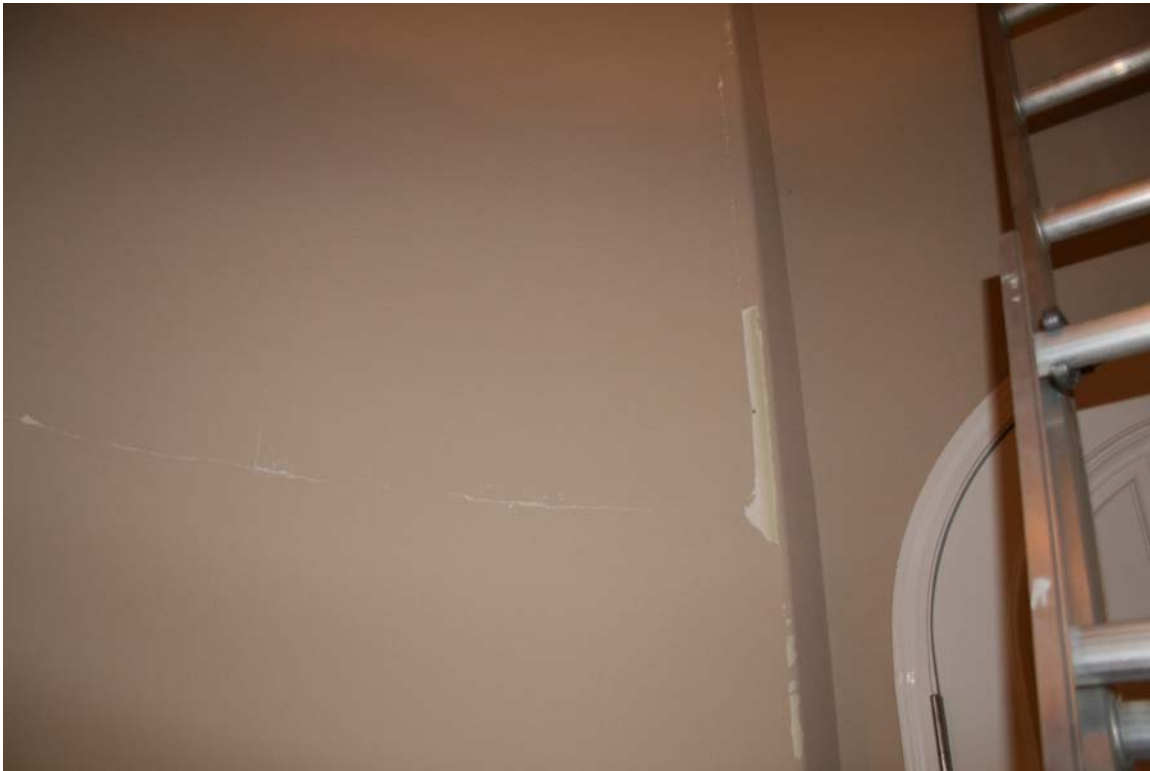
Figure 12 Cracking of plaster and paint in entryway of a home.
