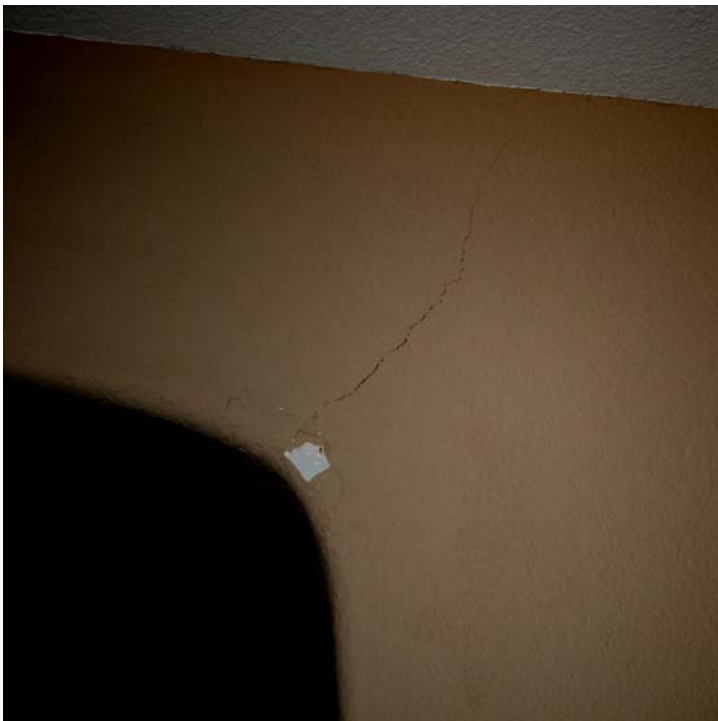
Figure 15 Common position of diagonal cracks near top corner of entryways or openings.
