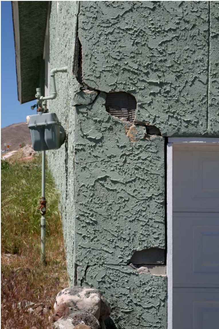
Figure 17 Close up of cracked stucco from rocking motion of house in figure 16. Note the gas meter that apparently flexed along with the motion successfully.
