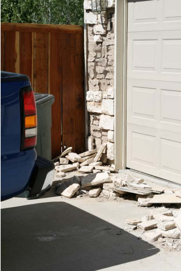
Figure 21 Detail of dislodged and damaged decorator rock.
