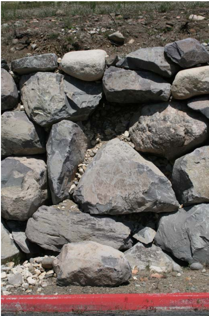
Figure 23 Boulder that fell out of the middle of a rockery wall (boulder is laying on the ground in front of the wall, closet to the red curb).
