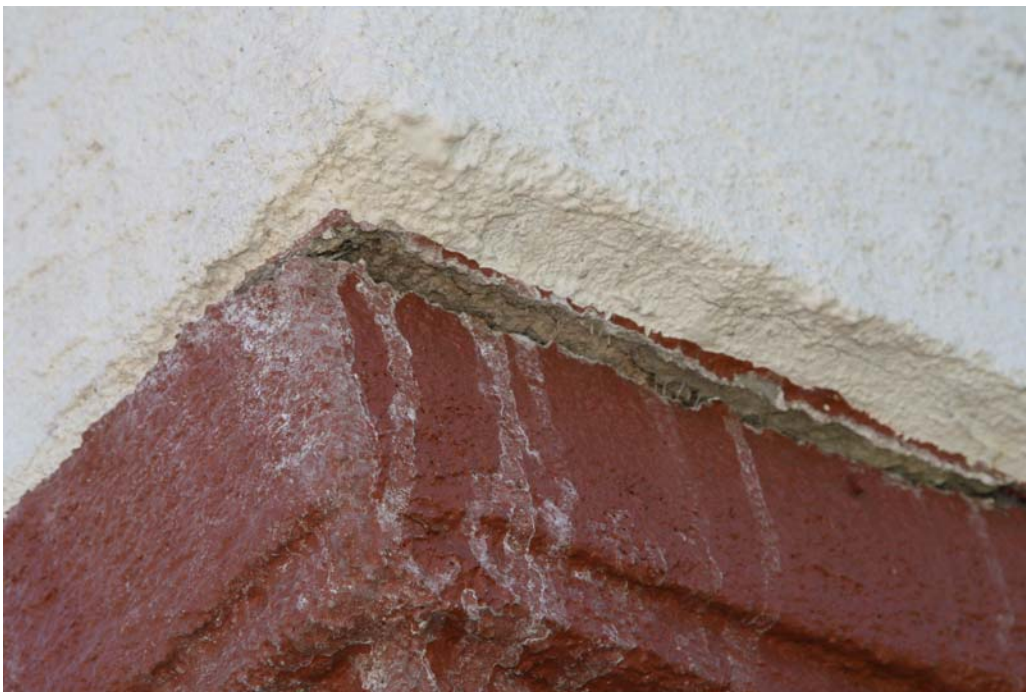
Figure 26 Top of pillar shown in figure 25 displaced from top about 2/10 th s an inch.
