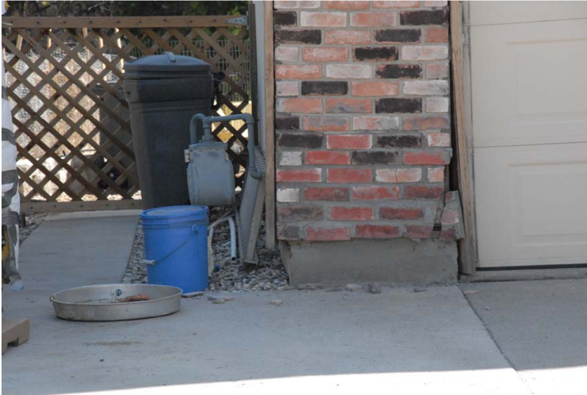
Figure 24 Corner of garage wall displaced to left off its mud sill. The gas meter handled movement successfully. (Photo by John Anderson)
