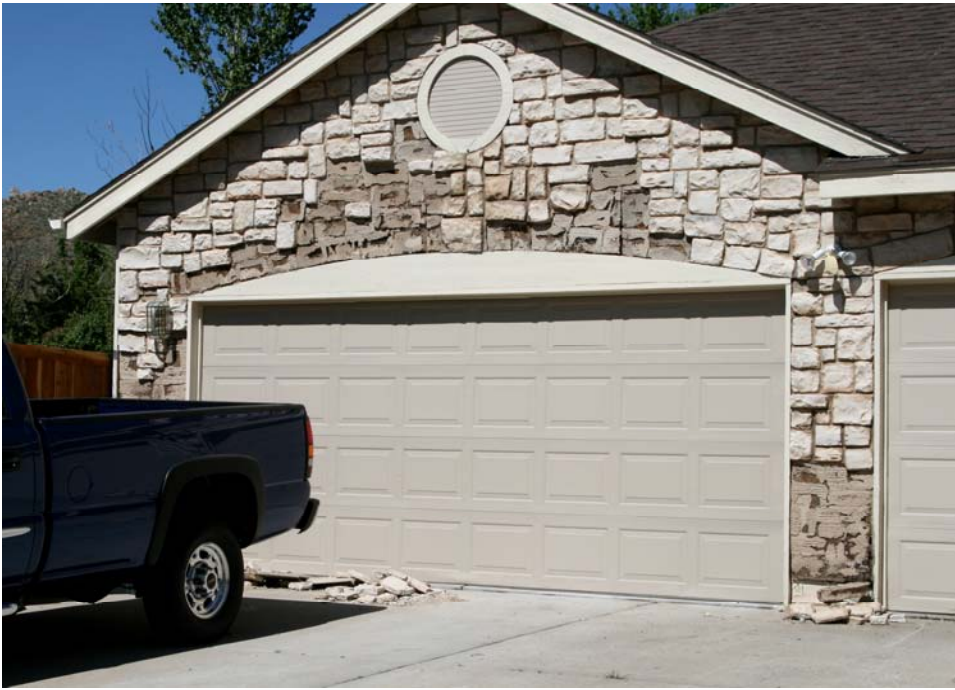
Figure 20 Decorative rock was popped off the garage, caused by the movement and distortion of the garage during shaking.
