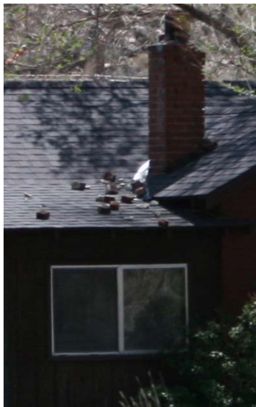
Figure 42 Several bricks were thrown from this chimney near Mogul.
