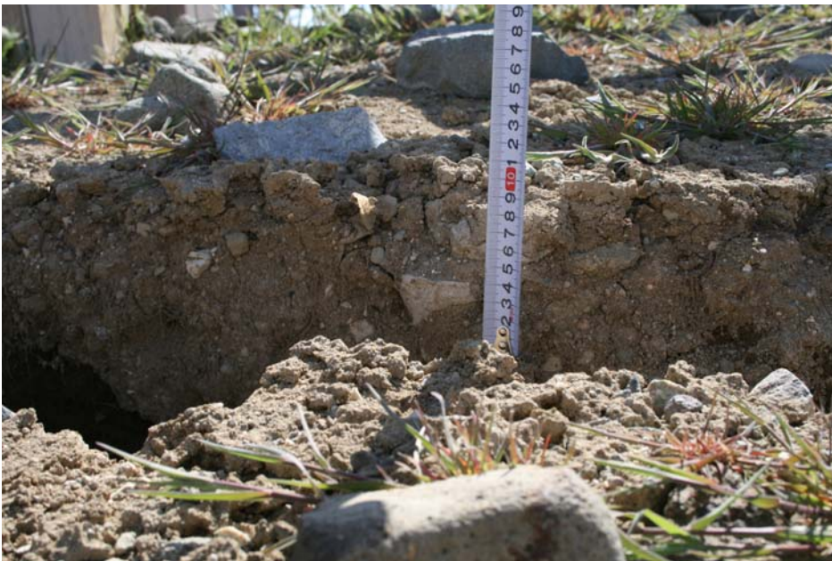
Figure 29 Approximate settlement of fill adjacent to the rockery wall in figure 28; scale is in centimeters. Here the scarplet is about 4 inches (10 cm) high.
