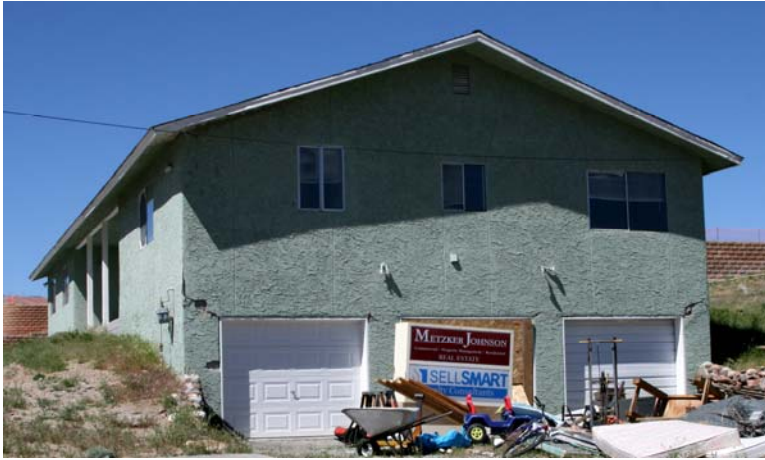
Figure 16 This house was rocked back and forth, cracking the stucco in the lower part, near the top of the three garage door openings. The slope created a small vertical irregularity in the structure and the garage door openings acted as a relatively soft first story.
