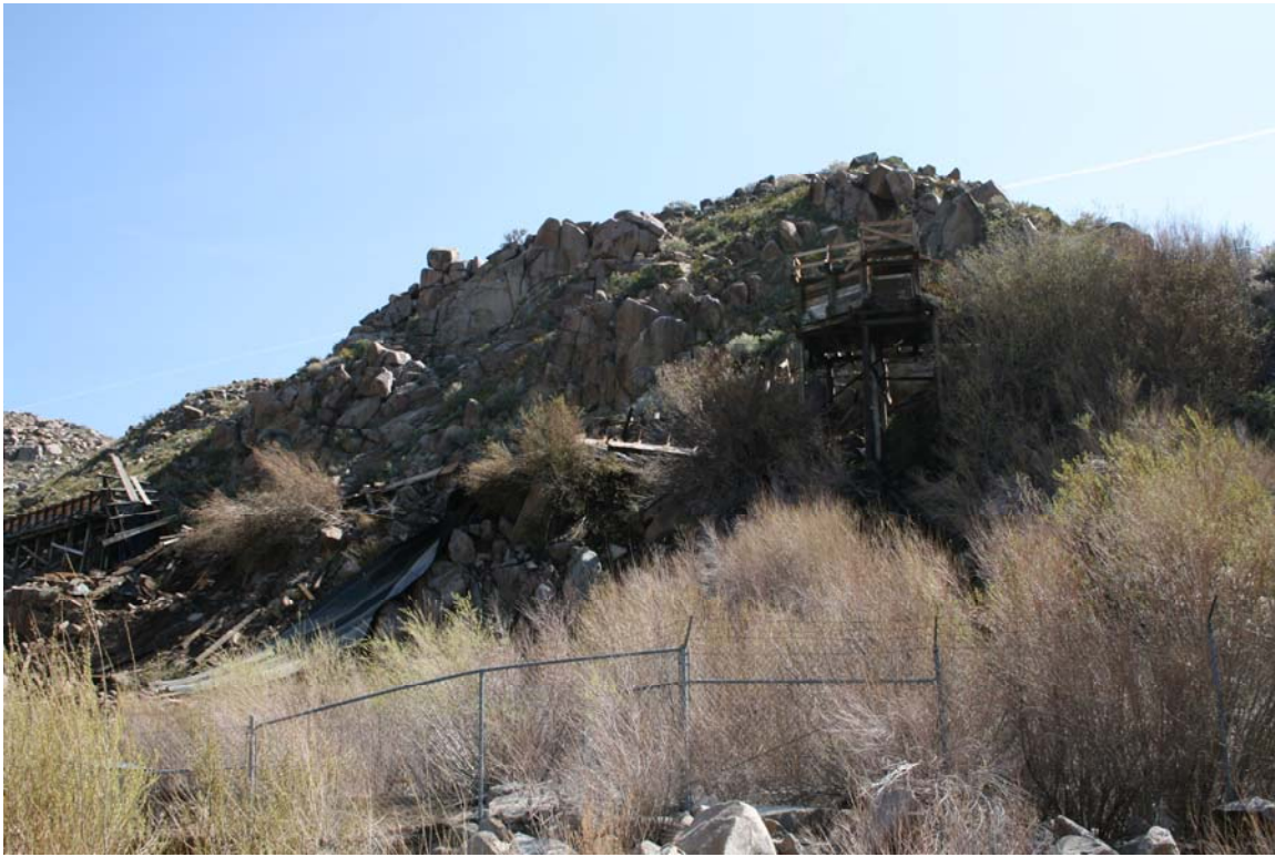
Figure 45 Rock fall damage to water flume.
