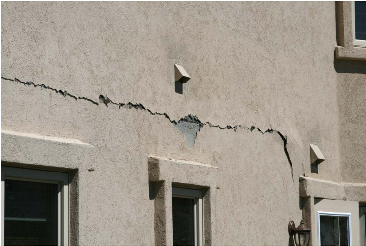
Figure 18 Horizontal fracture in stucco exterior of a house.
