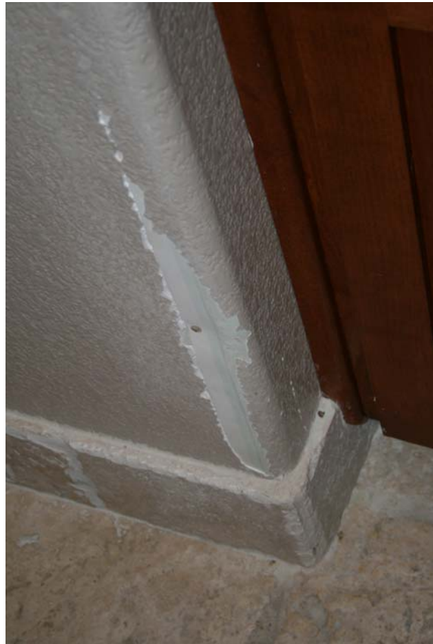
Figure 13 Cracking and chipped paint was broken away from the seam from rocking motion of a house.
