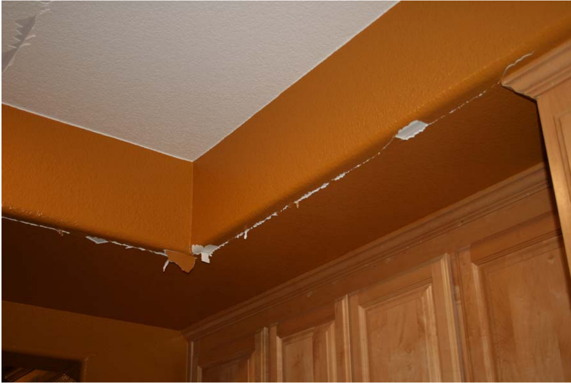
Figure 14 Damage to plaster and paint along seams in a kitchen from rocking motion of house.
